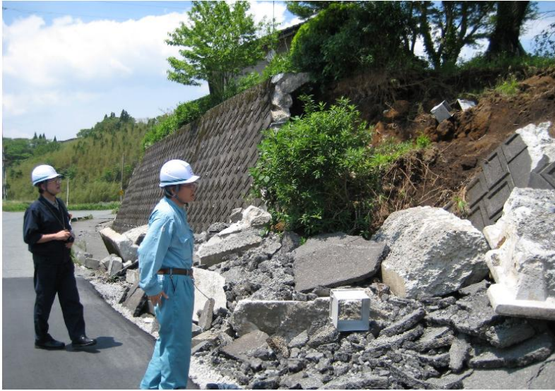
(a)練積み擁壁崩壊
